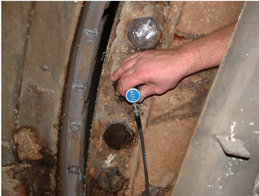
Fig. 6: fronts of the bolts are clean for UT
